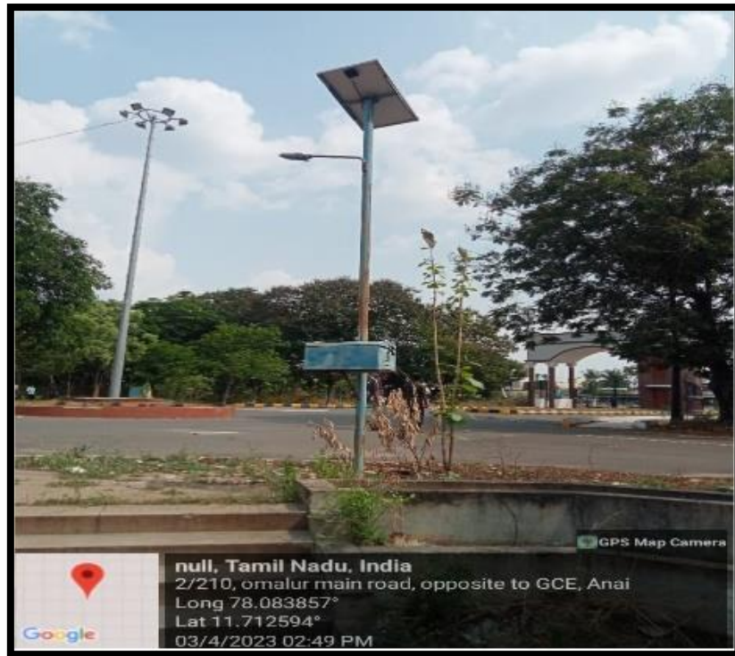
Figure 1: Solar energy-based street lighting system
