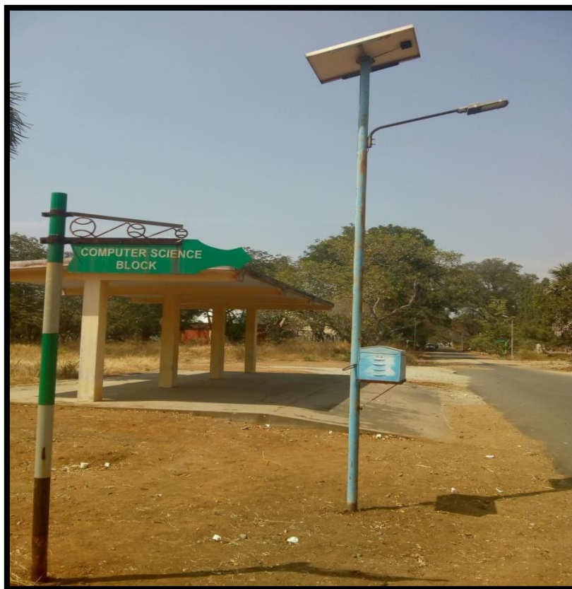
Figure 2: Solar energy-based street lighting system
